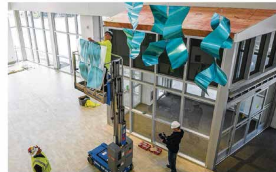
Local artist and architect Terry Welker hangs his commissioned piece in the new Five Rivers building at 721 Miami Chapel Road on Saturday. The new building, to open in mid April, will permanently display the work of many local artist. SARAH BENNETT / CONTRIBUTED
